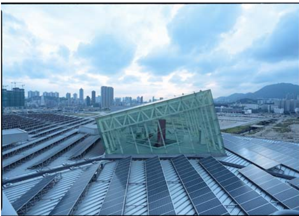
Fig. 1: BIPV installation in EMSD Headquarters
