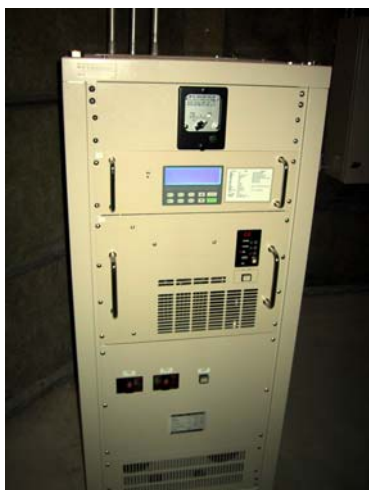
Figure 7: Power Conditioning Unit
