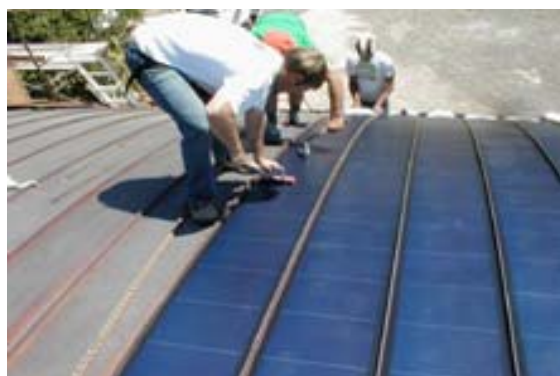
Figure 1: Flexible Amorphous Thin-film PV Panels installed on curved surface (Photo source: NREL)
