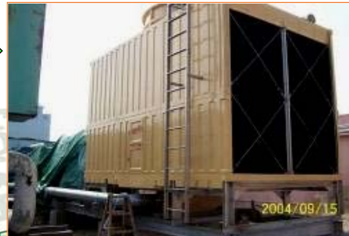
Water-cooled A/C system
