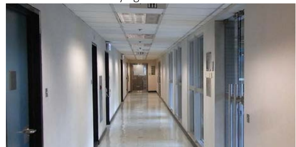
Figure 4 – Unrequired lighting for corridor without occupancy
