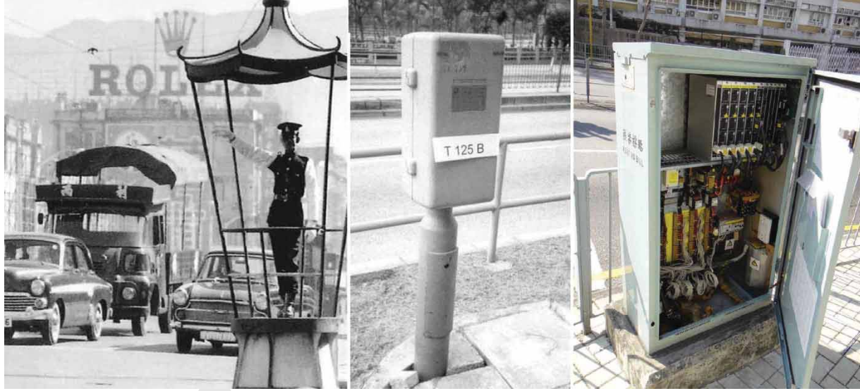
Figure 5. Traffic pagoda (left), early type of traffic signal controller [2] (middle) and latest ATC-connected controller (right) maintained by EMSD.
