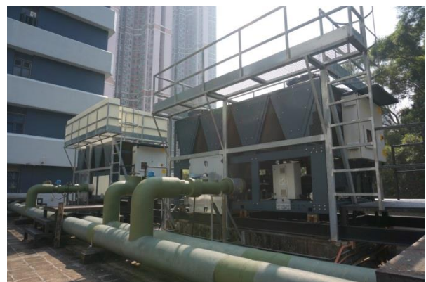
Fig. 9 New Air-cooled Oil Free Chillers at a Disciplinary Building
