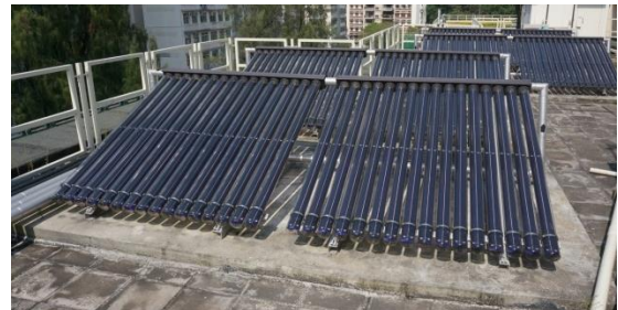
Fig. 8 Solar Water Heating System
