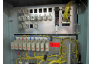
Obstruction Switch installed in the Control Panel
