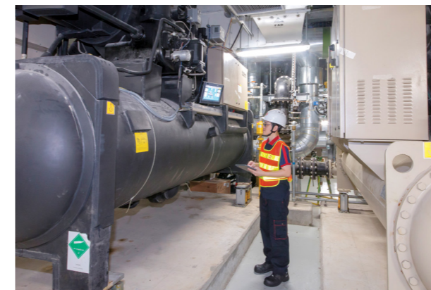
機電署正為庫務大樓的製冷機安裝人工智能優化系統安裝工程，透過數據分析提升能源效益；同時，我們致力在大樓內採用更環保的消防滅火劑。Aiming to enhance energy efficiency through data analysis, the EMSD is currently arranging installation of AI optimisation system for the chiller at the Treasury Building. Meanwhile, efforts are underway to adopt greener fire suppressants throughout the facility.
