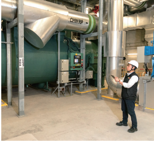
為北廠內的製冷設備進行定期檢查和維修保養。 Regular inspection and maintenance of chiller equipment inside the North Plant.
