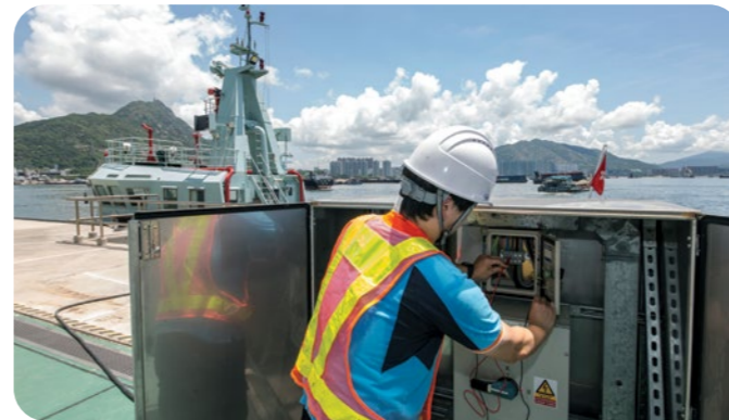
機電署負責為屯門滅火輪消防局的緊急發電機、低壓電掣房及防水閘等設備進行維修及保養，以確保設備運作暢順，並切合場地的特定需要。 The EMSD is responsible for the repair and maintenance of equipment such as the emergency generator, low-voltage switch room and flood gates at the Tuen Mun Fireboat Station, ensuring smooth operation of the equipment and fulfilling the specific needs of the venue.
