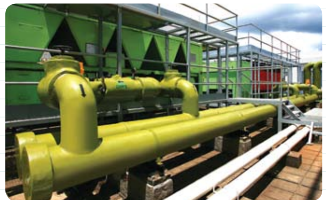
為威爾斯親王醫院更換製冷系統，令公眾人士有舒適環境接受醫療服務。 Replacement of chiller at Prince of Wales Hospital to ensure a comfortable environment is provided for the public to receive medical treatments.
