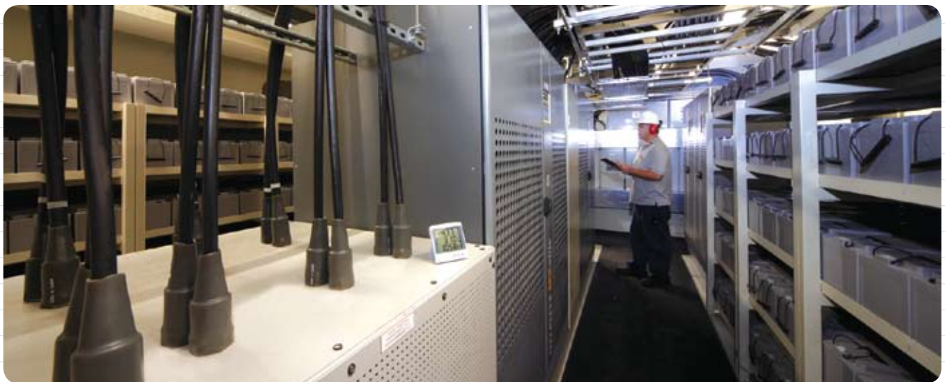
為廉政公署檢查一個雙重不間斷電源系統，確保系統在完成提升工程後可持續提供可靠的電力供應給電腦系統。 Checking a dual uninterruptible power supply system of ICAC to ensure the power supply reliability for computer systems after a major upgrade.
