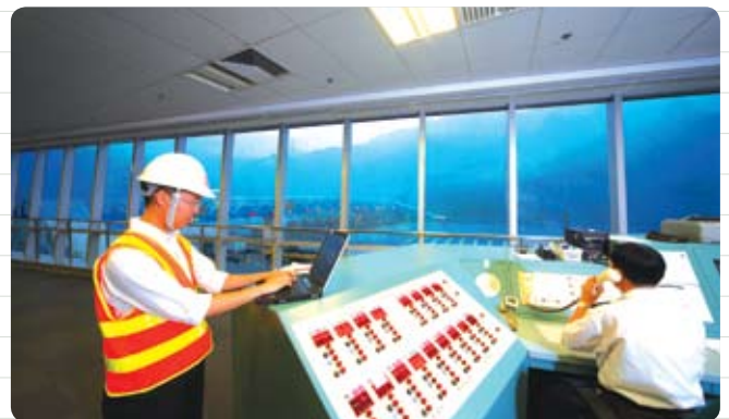
測試八號幹線控制中心的交通控制系統，確保交通流動暢順。 Testing the traffic control system at Route 8 Control Centre to ensure the smooth flow of traffic.
