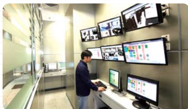
小蠔灣數據中心第一期落成，加強了我們爭取數據寄存新業務的能力。 The completion of Phase I of Siu Ho Wan Data Centre enhanced our ability to capture new business in data hosting service.
