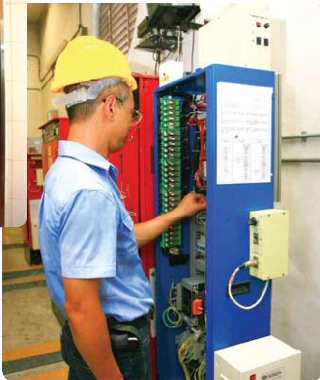
在已婚警察宿舍安裝具電力再生功能的升降機。 Newly installed lift with power regenerative feature at Police Married Quarters.
