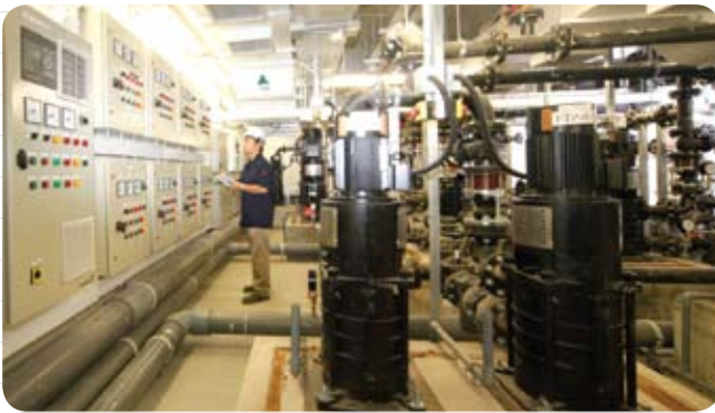
在羅湖懲教所為食水供應系統進行檢測，確保系統正常運作。 Inspecting the fresh water supply system at Lo Wu Correctional Institution to ensure the system operating in normal condition.
