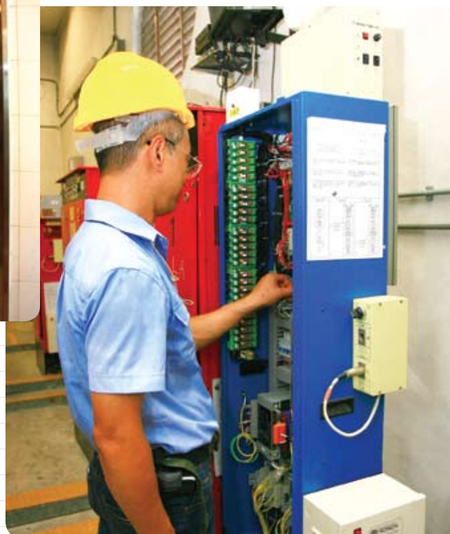
在已婚警察宿舍安裝具電力再生功能的升降機。 Newly installed lift with power regenerative feature at Police Married Quarters.
