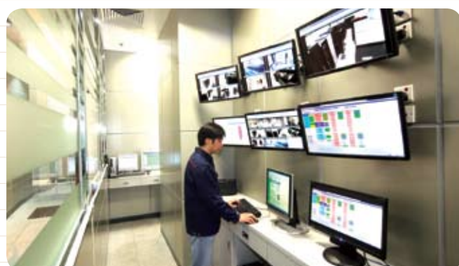
小蠔灣數據中心第一期落成，加強了我們爭取數據寄存新業務的能力。 The completion of Phase I of Siu Ho Wan Data Centre enhanced our ability to capture new business in data hosting service.
